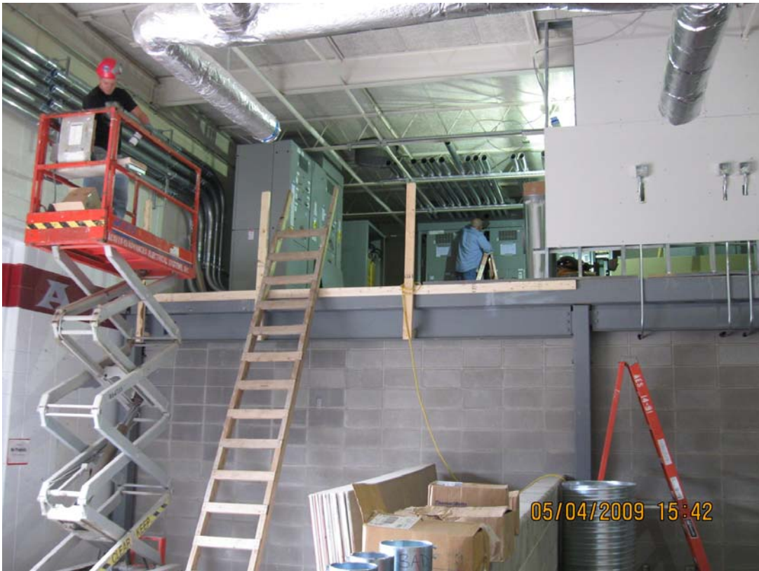
Unit G, Mechanical Room
