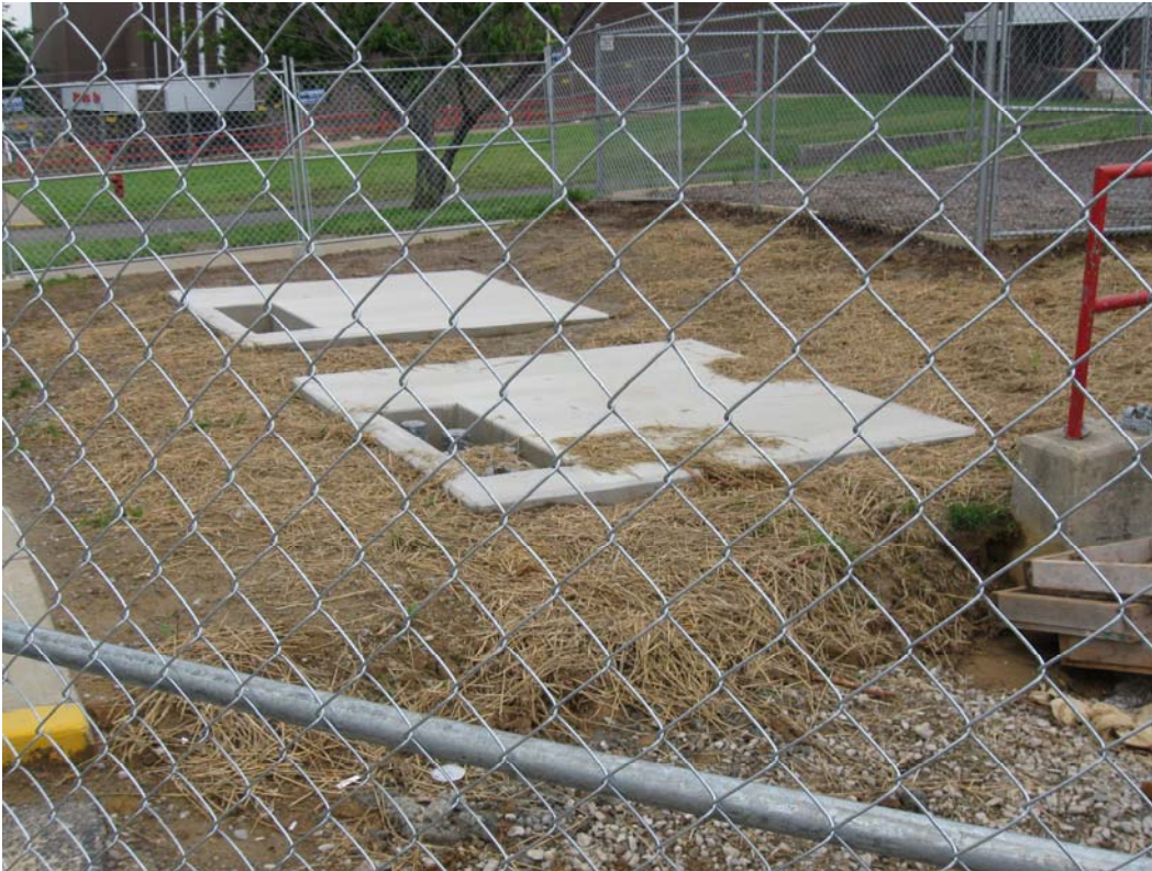
New Transformer Pads
